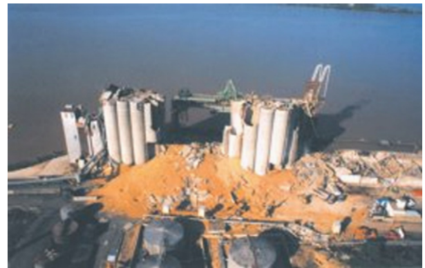
Fig. 3. The Blaye accident (1997). After a series of dust explosions a large number of silo cells were totally destroyed.
